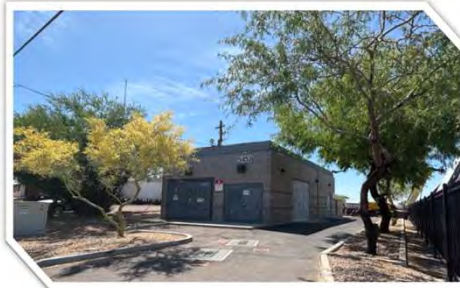
Traction Power Substation
